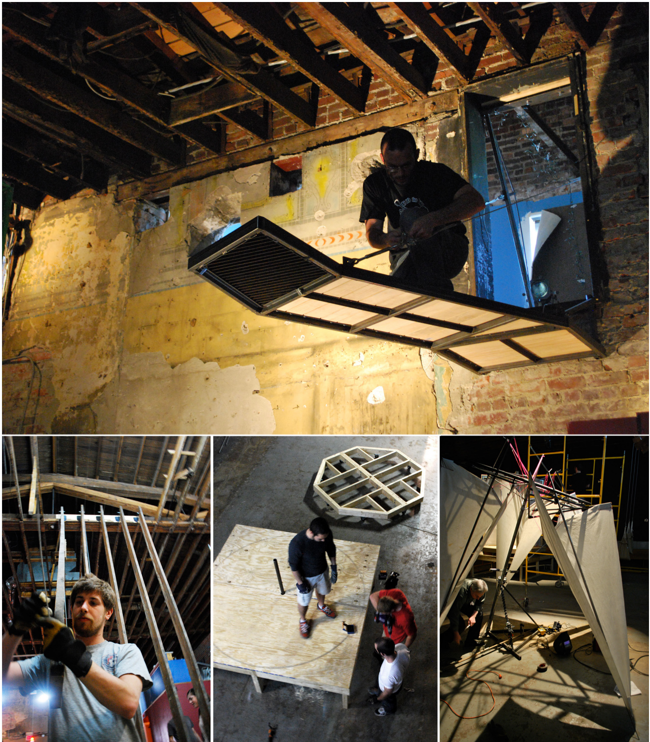
Figure 2: Architecture students installing their work in the theatre the week prior to the performance; clockwise from top: The "Perch" by Paul Reynolds; the "Choppa" by Jay Weeks and Austin Lucari; the "Beater" by Eric Jensen and Ben Greenberg; and "Strata" by Mark Vanden Akker, Brad Wanek, and Luke Haas
